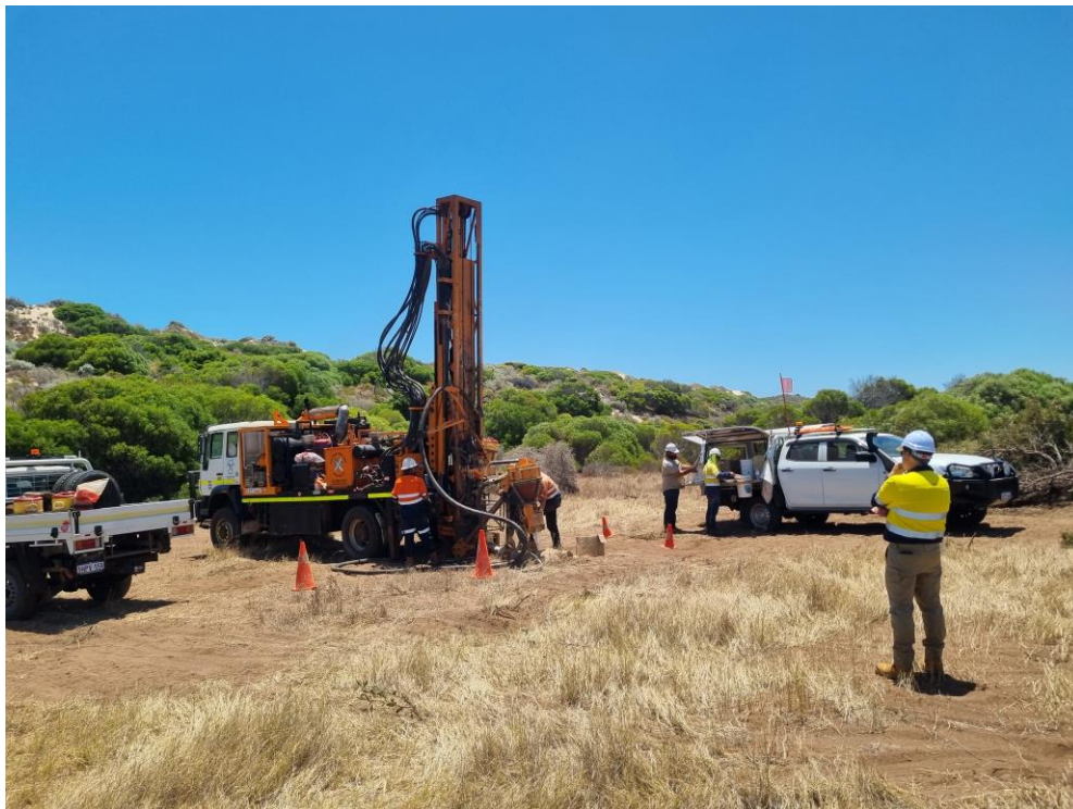
Figure 1: Maiden Drilling underway at the Red Hill Project with HVY Director Greg Jones observing.
