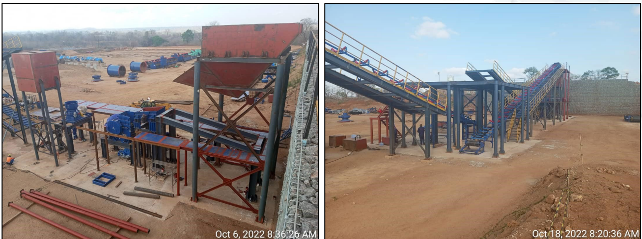
Figure 1: Mechanical installation of the crushing circuit (left) and Conveyors 1,2 & 3 (right). *Note that conveyor belting will be installed closer to commissioning.
