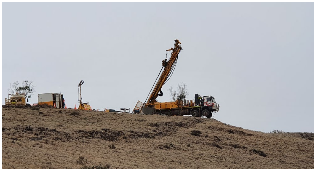
Figure 3. Iron Peak Drilling in difficult topography with outcropping magnetite (black) in foreground.
