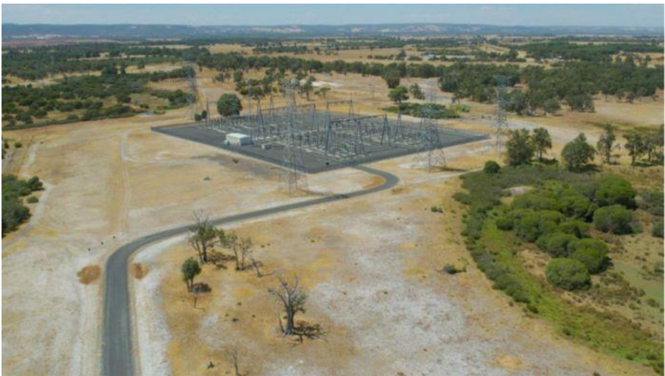
Image 2: Landwehr Terminal – 33/330kV
