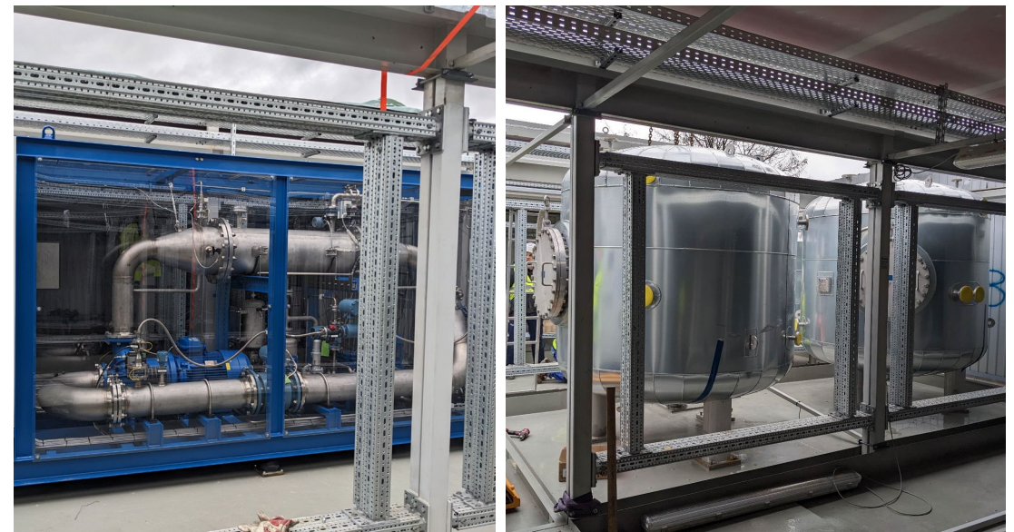
Demonstration Plant (LP & HP)
