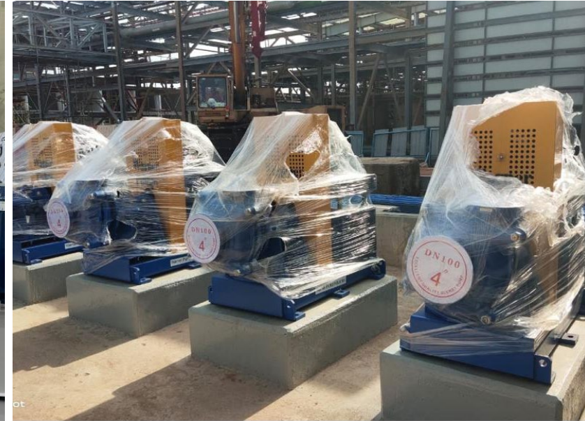
Sulphate removal pump
