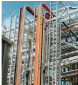
MARBL JV Kemerton Lithium Processing Plant – SCEE Electrical Over $100m
