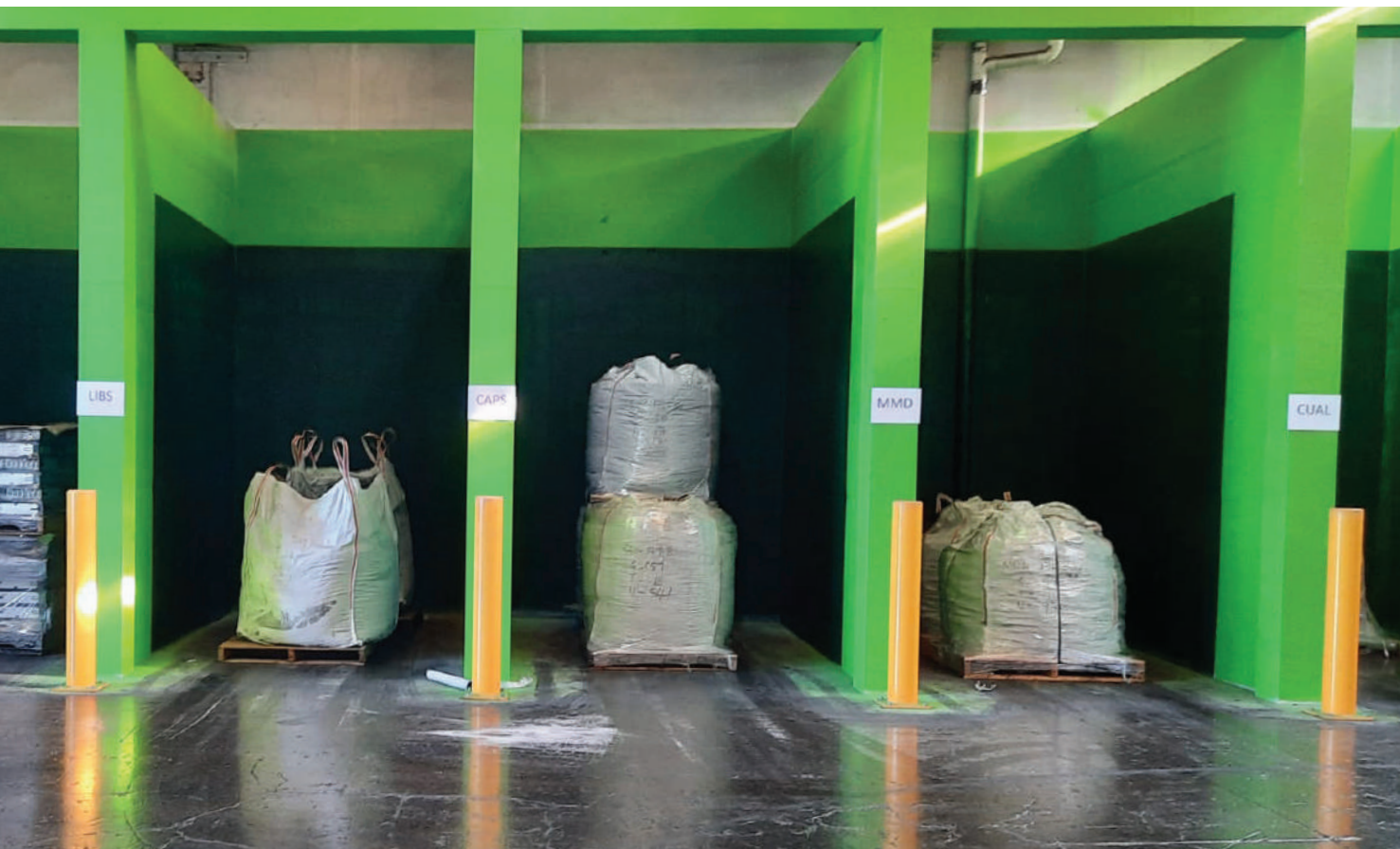
Firewalls at Envirostream's Campbellfield Facility.
