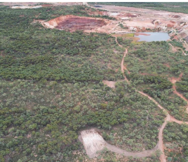
Figure 3. Clearing Drill pads yesterday for drilling to start, in the background is one of our existing pits
