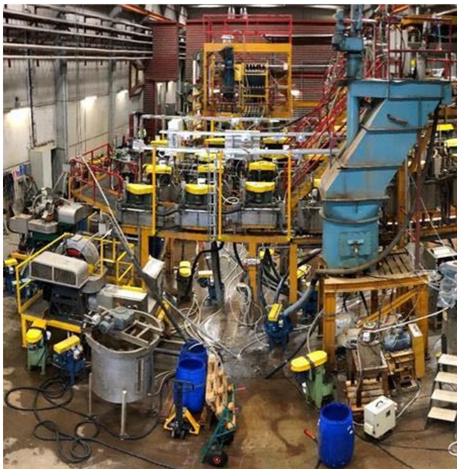
Figure 4.1.2: Overview of Pilot Plant including Magnetic Separators (bottom left), Lamella Thickener (right), and Flotation Cells (middle)
