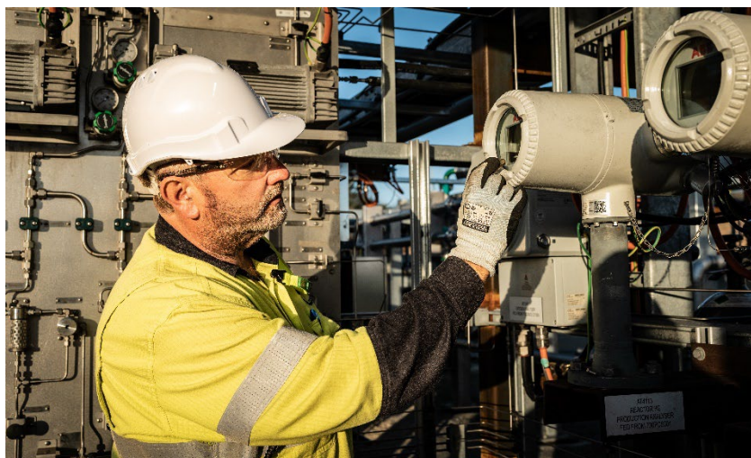
Equipment checks during flow test at the CDP plant, WA Australia
