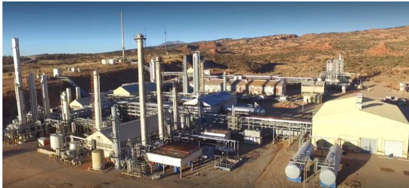
Figure 4: Paradox Resources "5.5 Nines" Lisbon Valley Gas Processing Plant.
