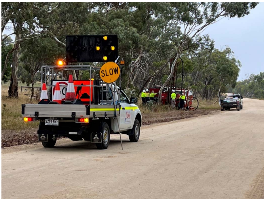
Image 2: Roadside Drilling Team on Bangham Road south of Bordertown with traffic control management in place
