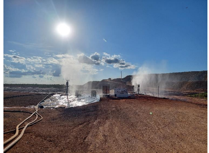
Figure 2: Evaporators installed for water management
