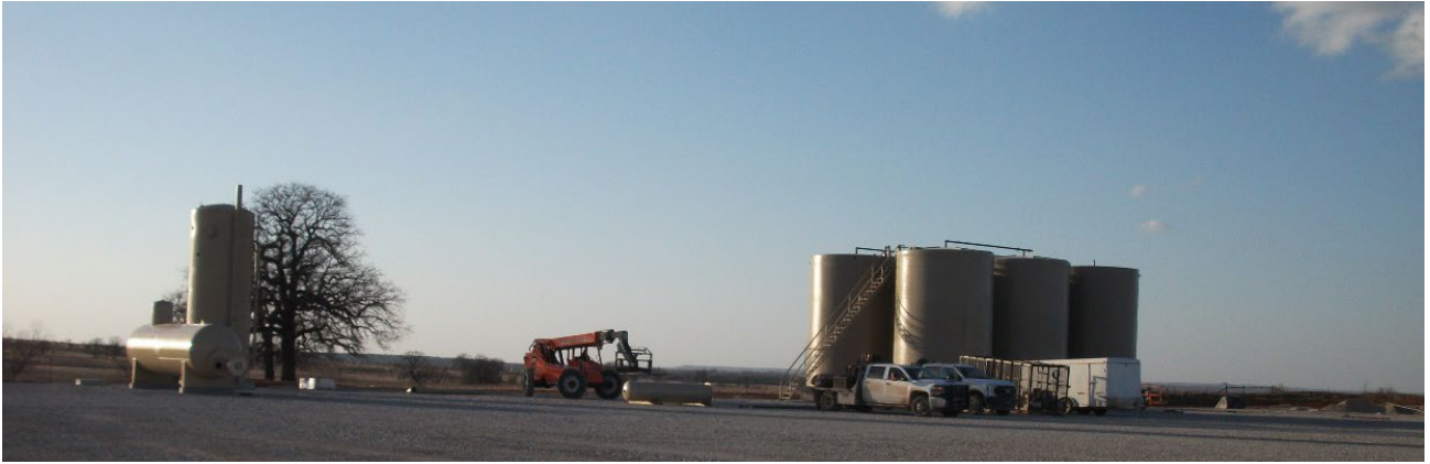
Figure 4. Rangers tank battery and separators
