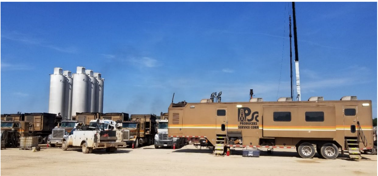
Figure 8. Producers Service Corp. (PSC) conducting multi-stage hydraulic stimulation operations on the Flames Well, Carter County, Oklahoma.
