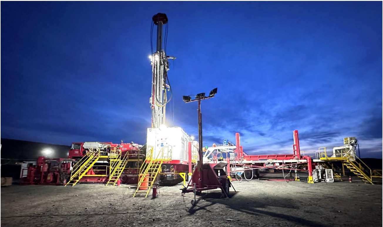
Figure 1 – Major Drilling Rig on location for the Lucky Fox - 1 pilot production well
