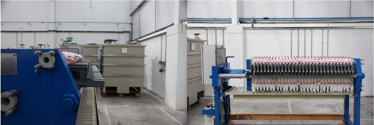
Figure 8: One of the Plate and Frame filter presses in position adjacent process reactor vessels.
