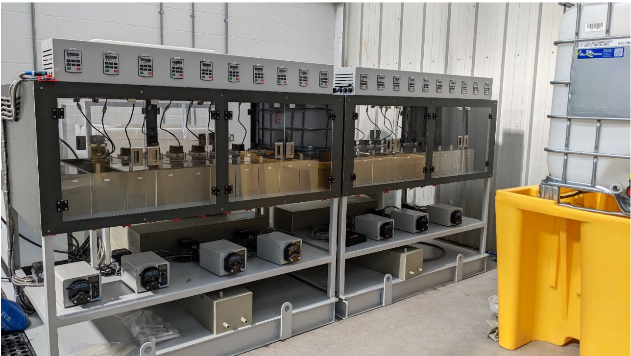
Figure 5: Mixer-Settler circuit installed.
