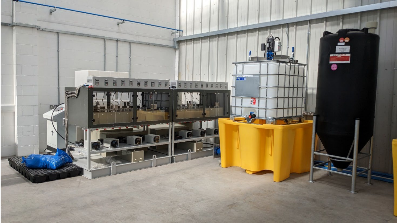
Figure 6: Mixer-Settler circuit installed adjacent to process reactor and settling tank.
