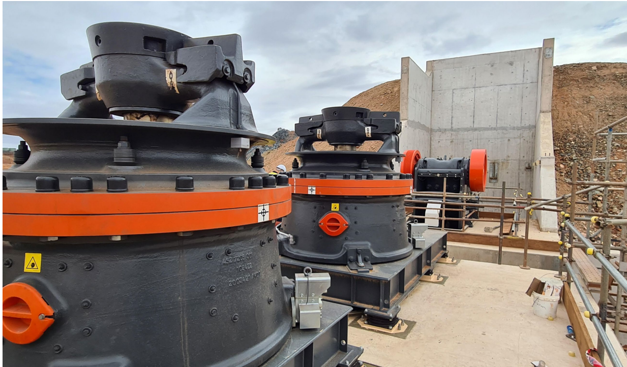
Figure 5: Crusher pocket including installed primary, secondary and tertiary crushers.
