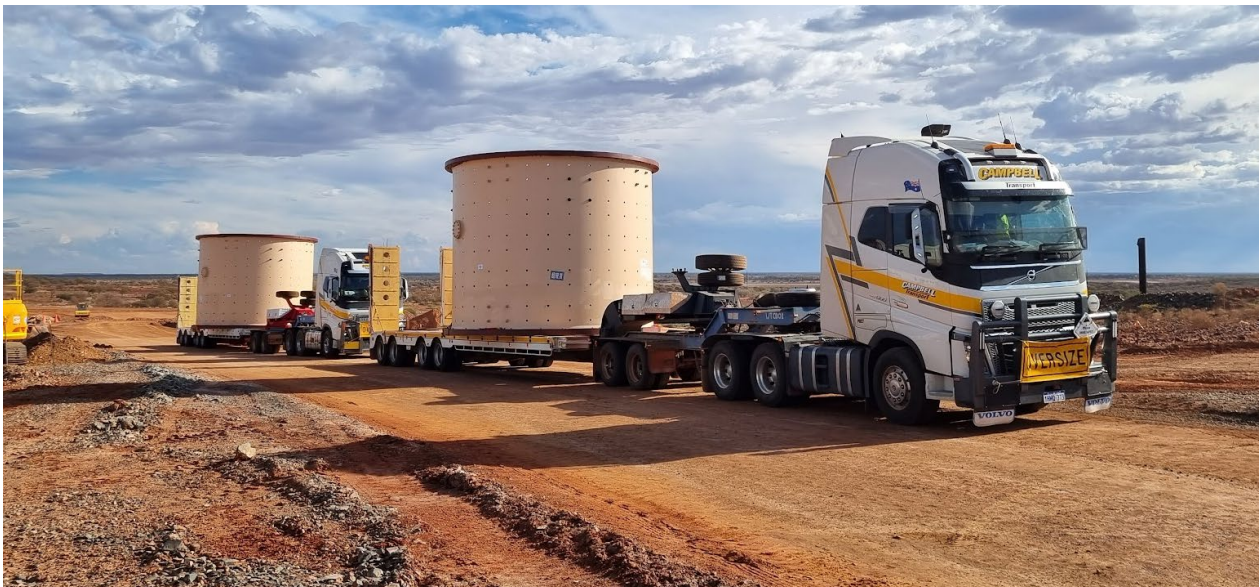
Figure 4: Ball mill arriving on site in March 2023 ready for installation, all critical long lead items have now been received on site significantly de-risking project delivery timeframes.
