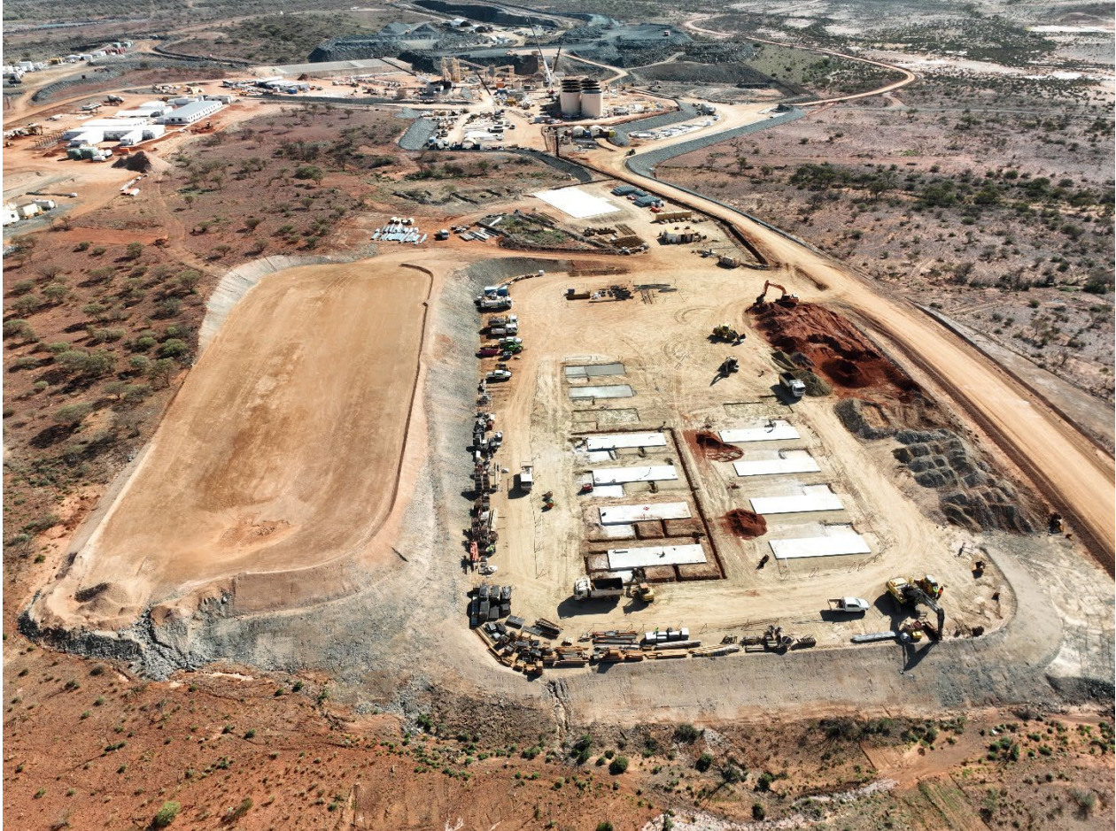
Figure 11: Power station construction as at 19 April 2023 including commencement of structural concrete for thermal generators.
