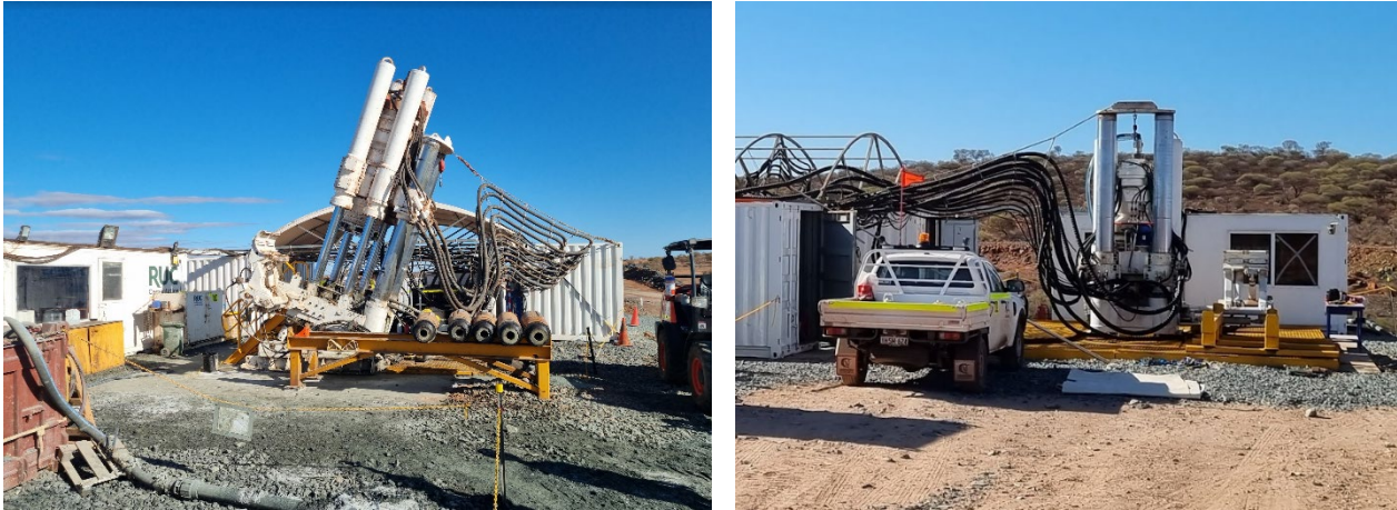
Figure 10: Bellevue site RUC raisebore drilling at the Northern escapeway rise (left); Second raisebore drilling rig at the Southern ventilation rise (right).
