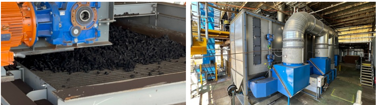
Photos (above): freshly extruded COLDry pellets enter the conditioning system (left) and wide view of the conditioning system, utilising waste heat from the co-located data centre.
