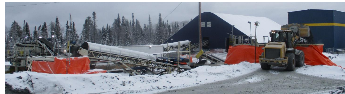
New crushing circuit
