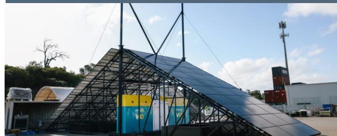
Ultra Power Systems has stand-alone power system at Second Fortune Gold Mine and will deploy to IGO's Silver Knight camp.
