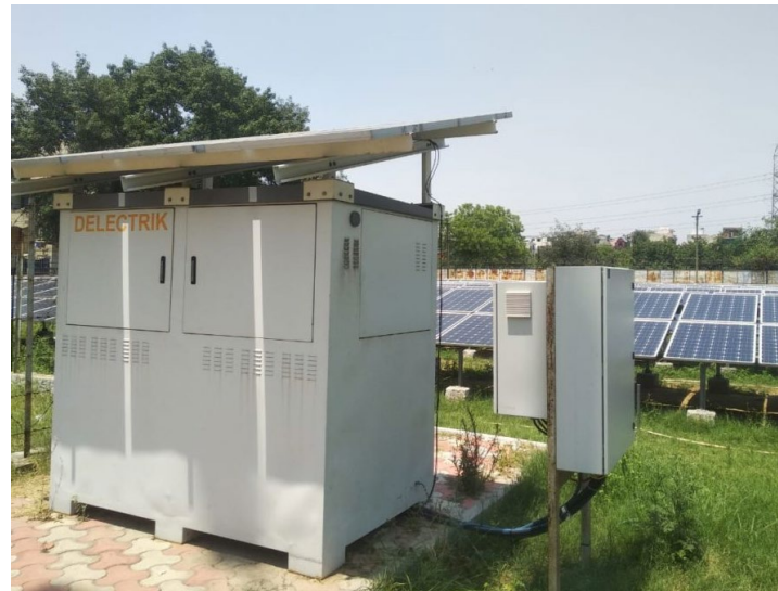
VRFB system installation by Delectrik Source: Delectrik Systems
