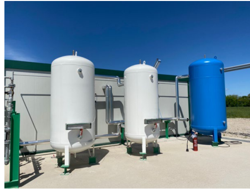
Figure 2 – Air & nitrogen tanks
