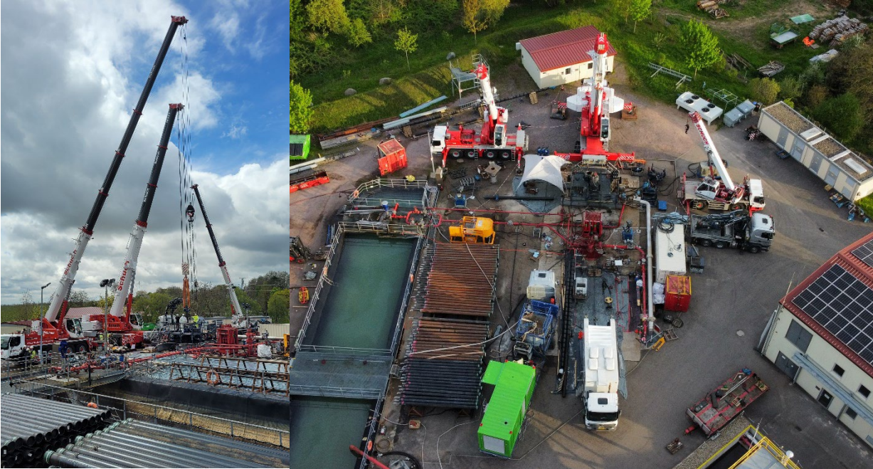
Cranes supporting Insheim pump change Aerial shot of Insheim whilst pump change in action.
