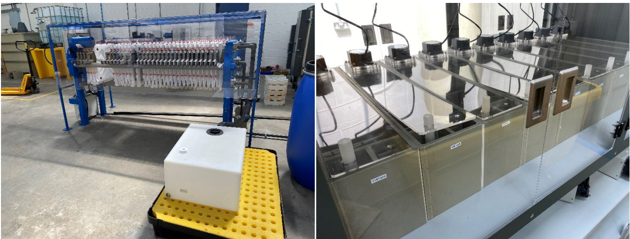
Figure 3: Safety screens installed around pressure filters and Solvent Extraction circuits.
