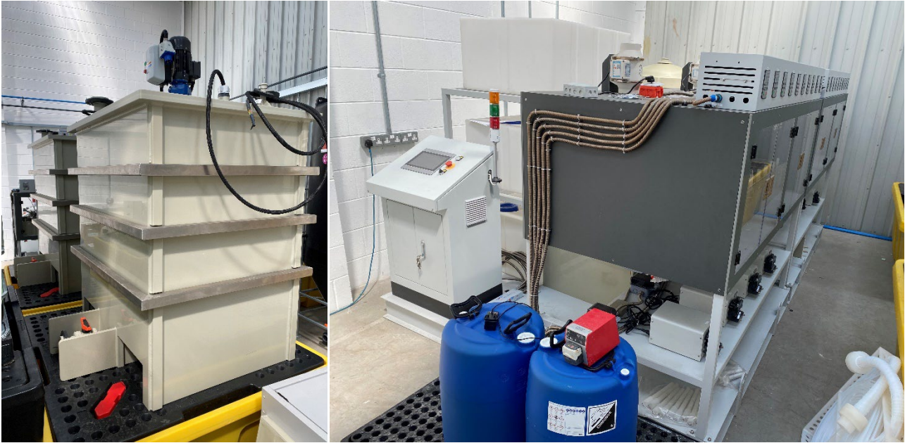
Figure 2: Leach reactors and Solvent Extraction circuit electrical installation completed, with process commissioning underway.
