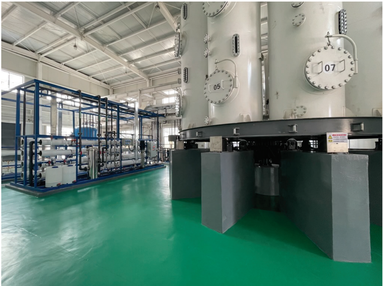
Figure 3: Lanshen DLE test facility in Xian, China
