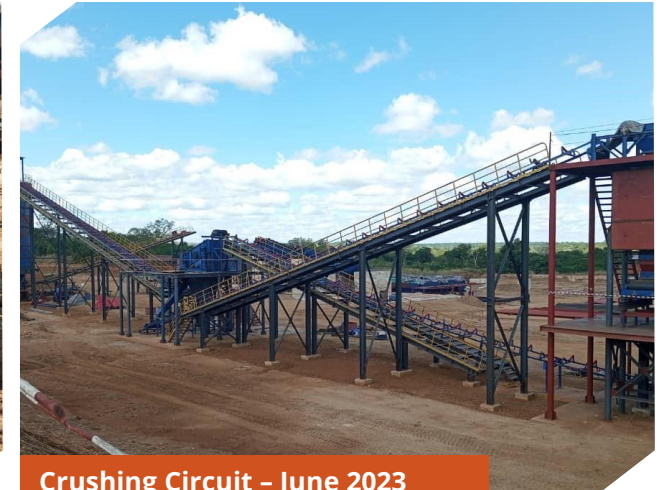
Crushing Circuit – June 2023
