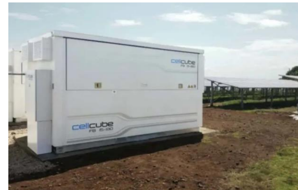
Plans unveiled for Australia's biggest vanadium flow battery and gigawatt factory. North Harbour Clean Energy backed by Aware Super and CellCube will build a 4MW, 16MWH VRFB for an industrial customer.
