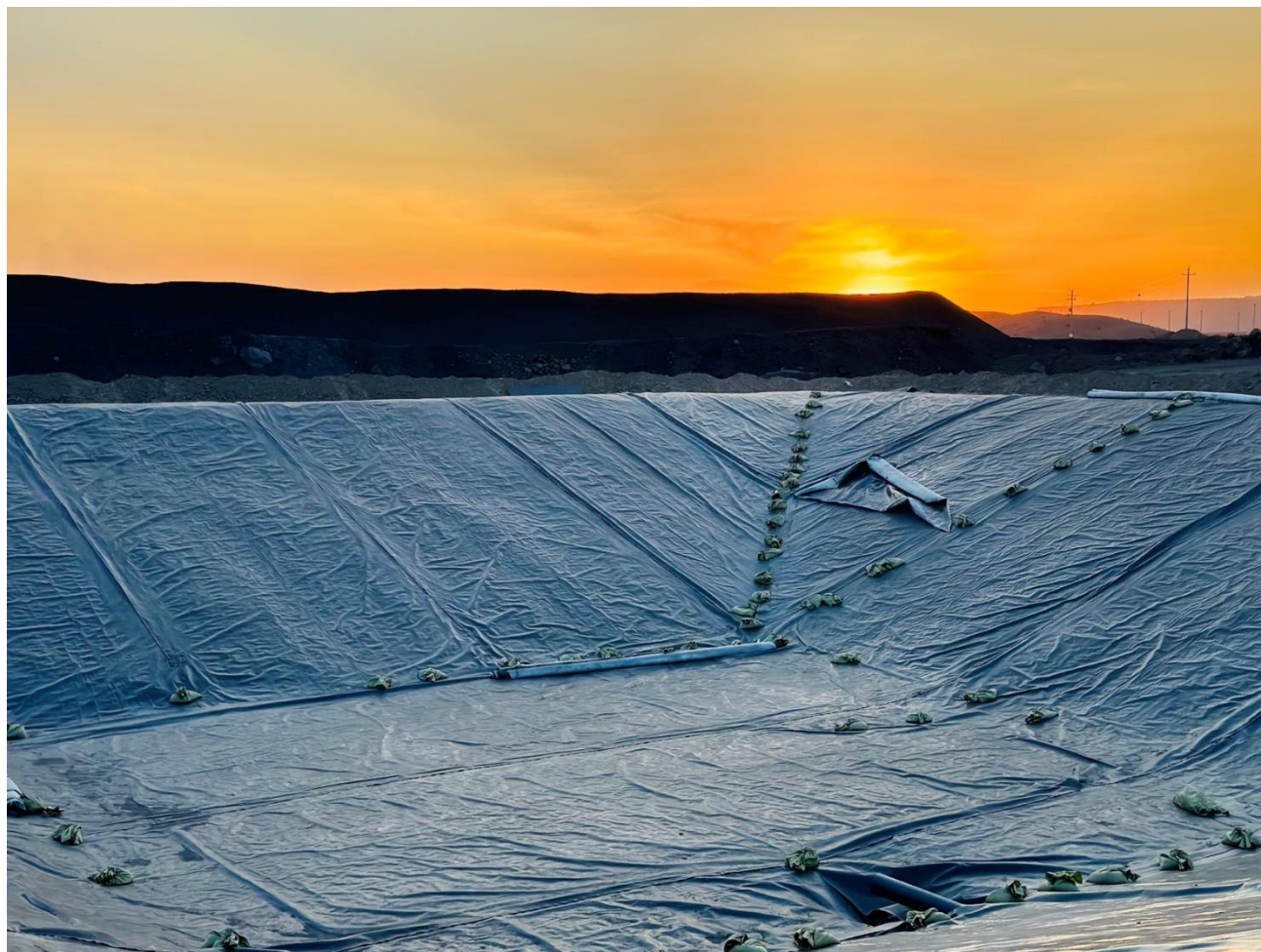
Figure 2 – Water handling facilities at the Gurvantes XXXV Coal Seam Gas Pilot Well Program
