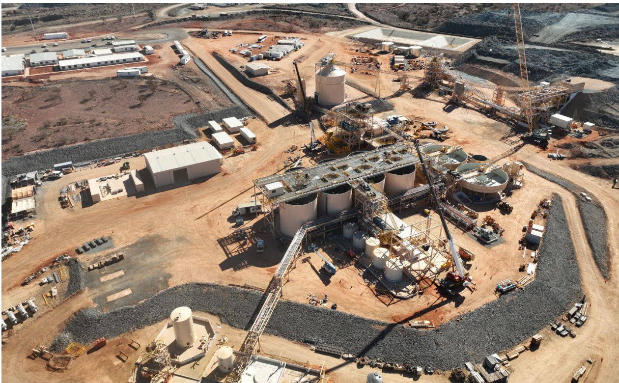
Figure 1: Progress shot of construction progress at the processing plant as at 16 July 2023.
