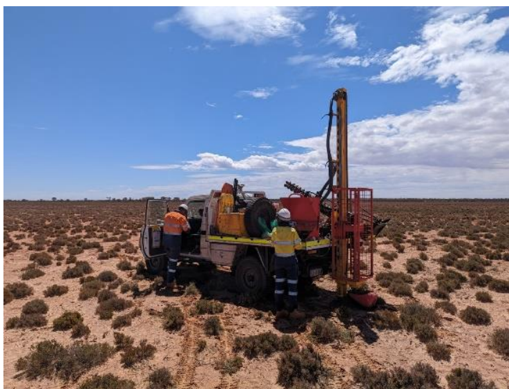
Figure 11 – Landcruiser mounted Auger Rig, with a depth capacity of 30m, was utilised with a 4-inch bit.
