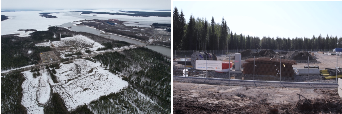
Figure 2 Land cleared at Refinery site at Luleå Industrial Park (L); electrical substation under construction (R).
