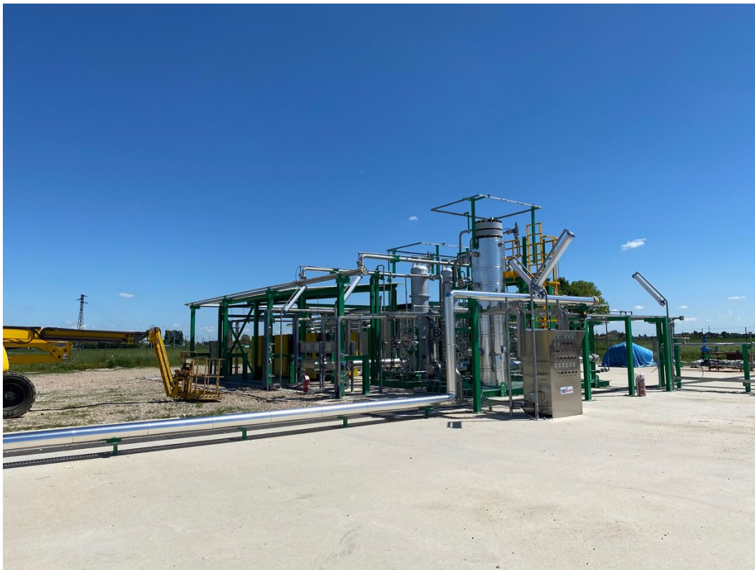
Figure 2: Podere Maiar – 1 Gas Plant
