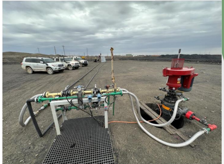
Completed Lucky Fox-3 coal seam gas well.
