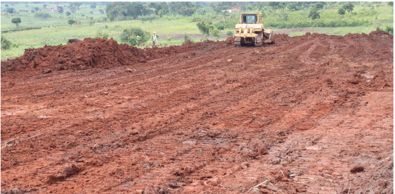
Figure 3: Demonstration plant earthworks progressing at the site of where the Makuutu Demonstration Plant Technical Facility will be located.
