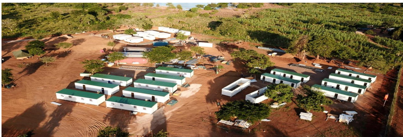
Above: Shankara Lodge facility, showing camp modules for TSK being assembled prior to transportation to site. The start of the 80-man camp is shown in the top left area of the photograph
