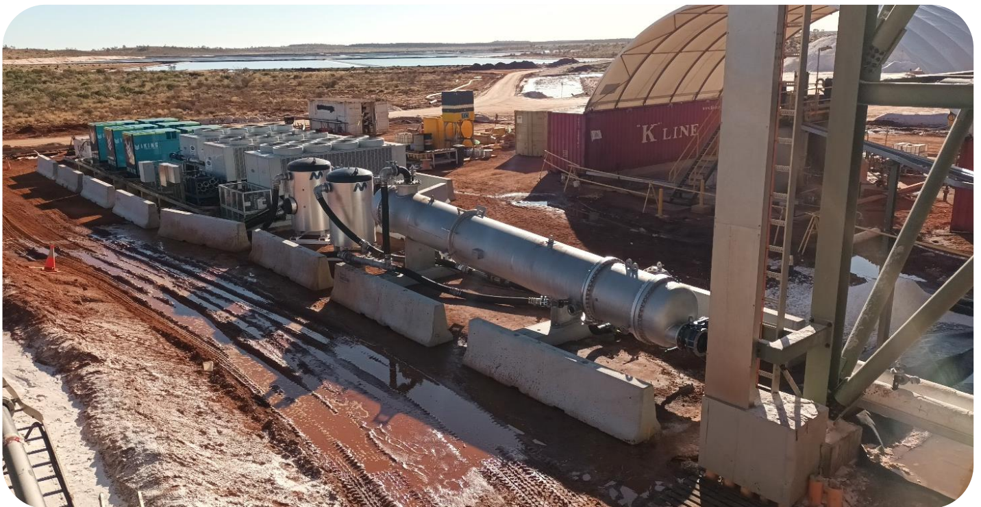
Second heat exchanger and equipment on site and tied into plant, July 2023
