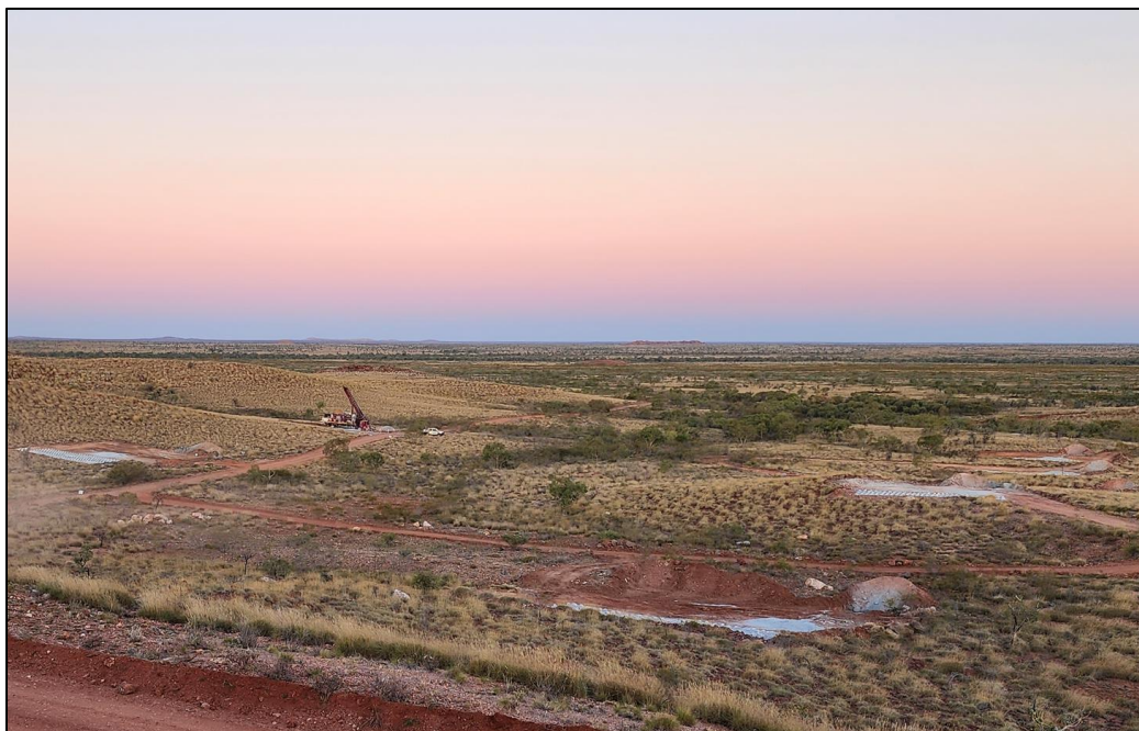
Figure 1 – RC drilling is progressing well at Tabba Tabba, with a second rig locked in to commence around the 10 th of August (view looking east).
