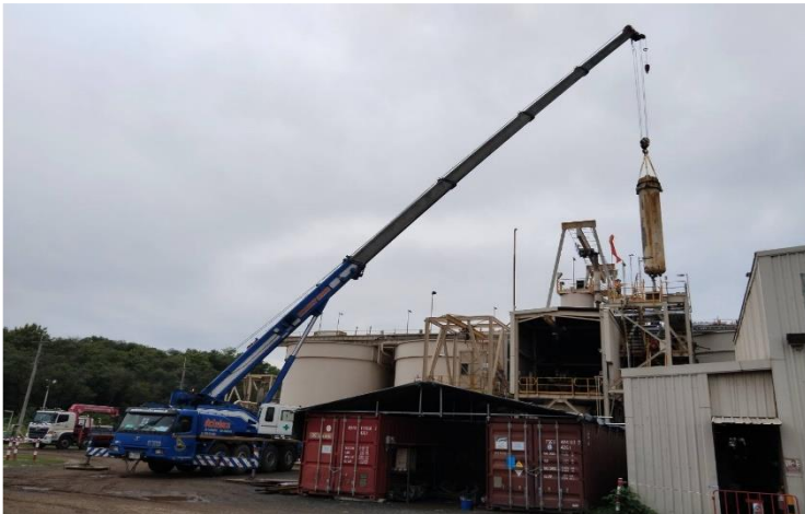
Plant #1 Overhaul Project: New grid mesh replacement (top left), solution tank removal for repairs (right), and acid wash column removal for repairs (bottom left).
