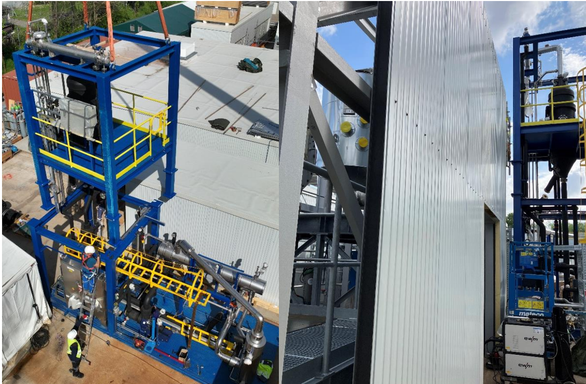
Figure 2 and 3. Crystalliser installation
