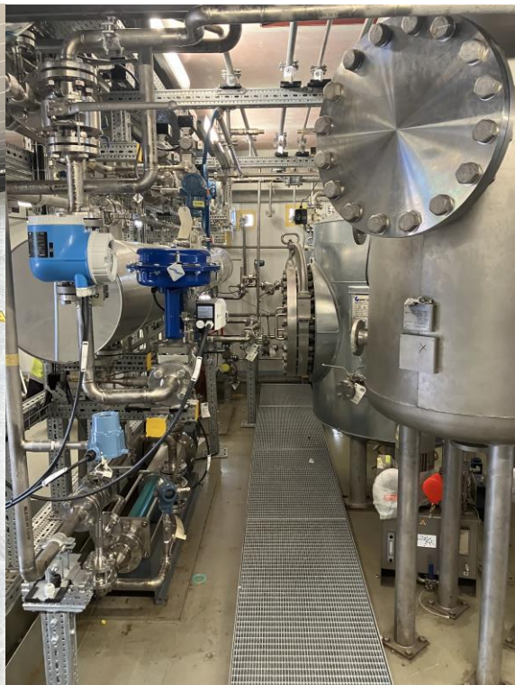
Figure 5. Brine Conditioning System
