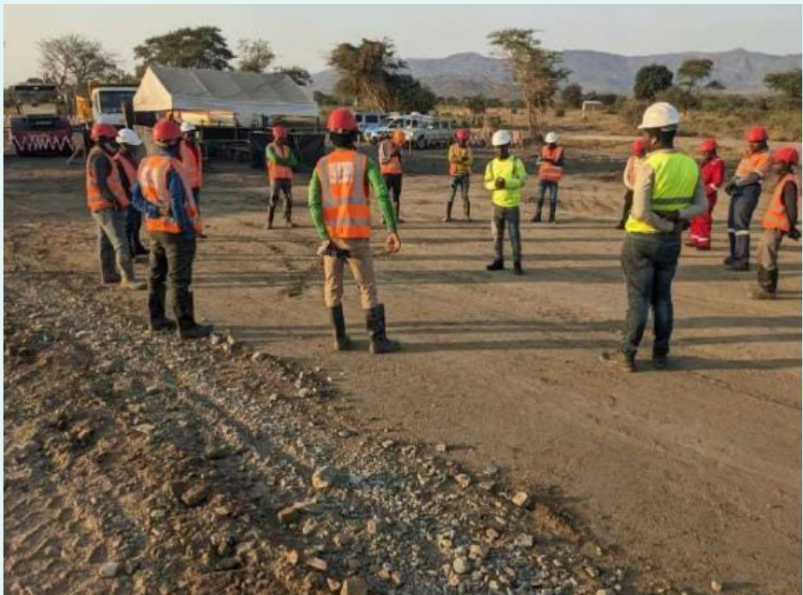
Construction of our Mbelele-1 and Mbelele-2 well sites are being carried out by our local civil engineering contractor.
