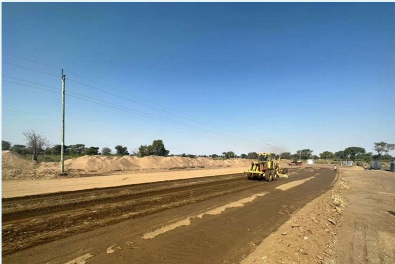
The Mbelele-1 site is on track to be ready by the end of August, well ahead of the rig's arrival in Tanzania. Mbelele-2 site is on track to be ready by early September.
