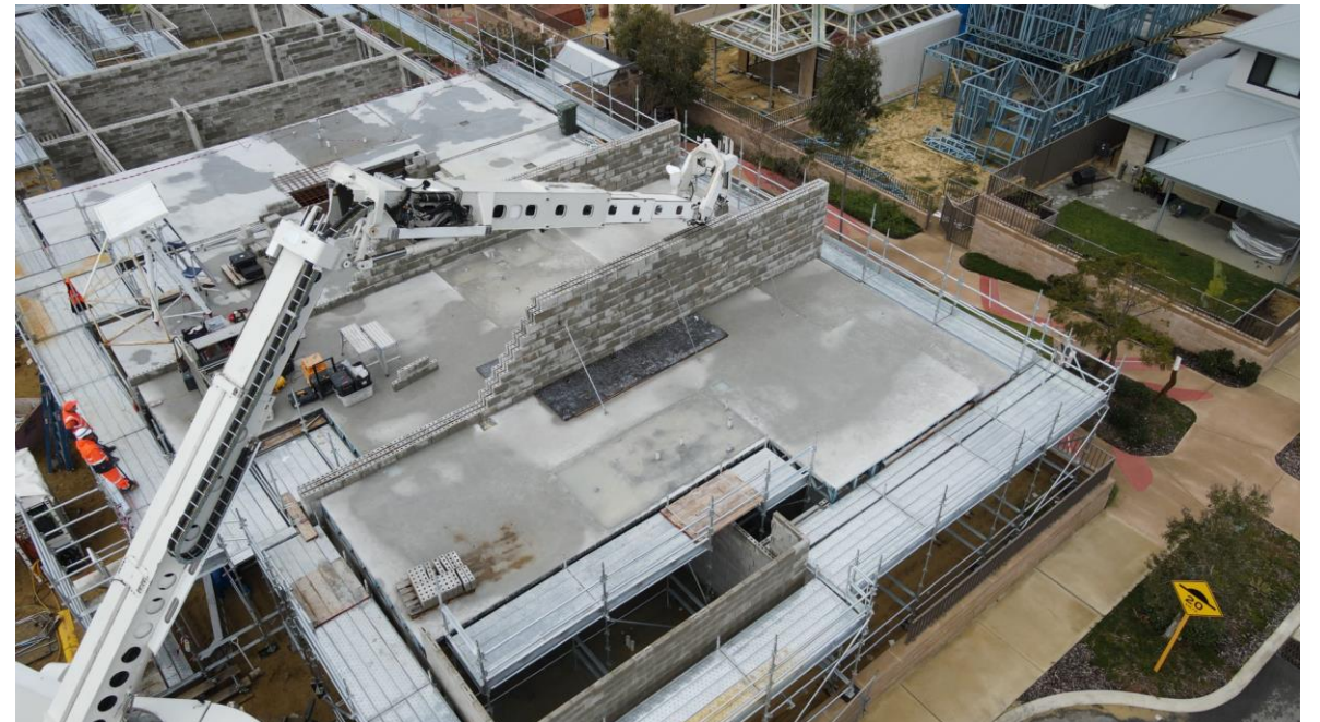
Final phase of works at Willagee sees blocks laid of second storey triple-leaf walls at the northern wing
