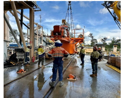
Figure 6 | Okvau Maintenance Personnel
