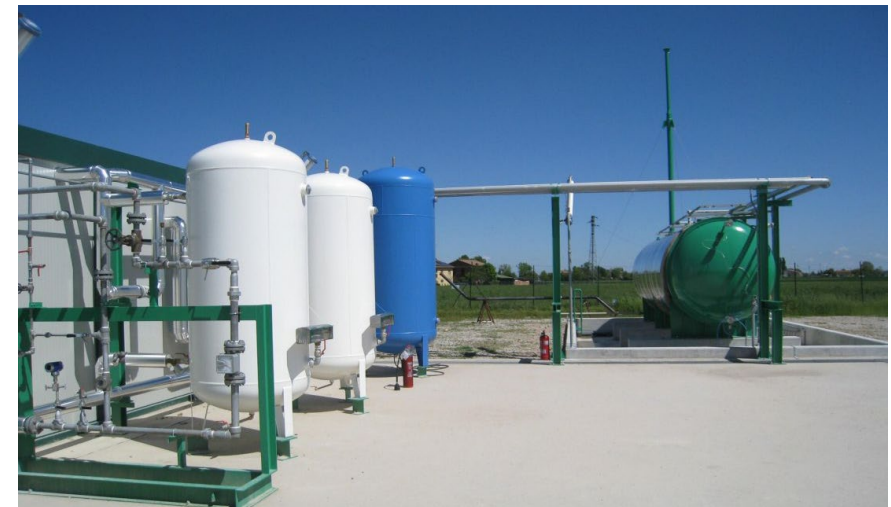
Picture: Nitrogen tanks at Podere Maiar – 1 well site
