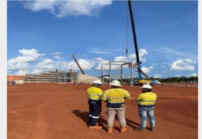
Structure for primary crusher discharge
