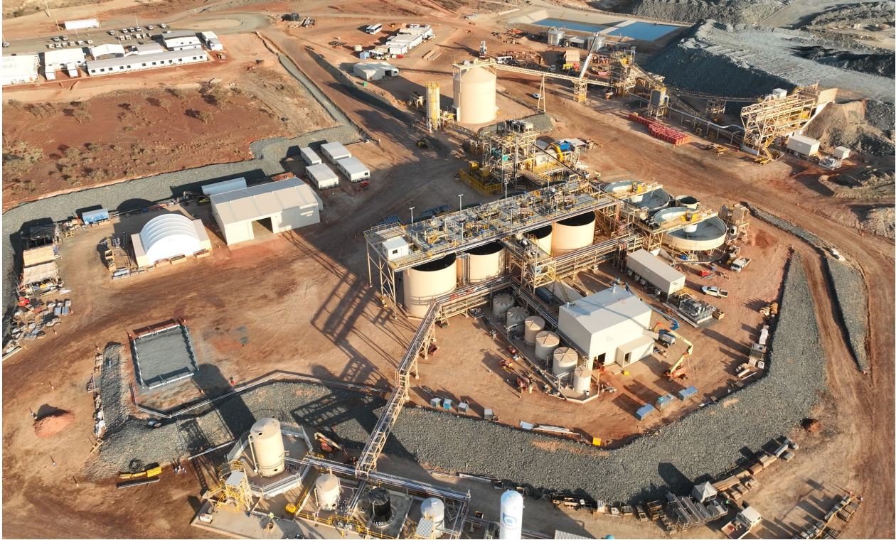
Figure 6: Construction progress on site at the Bellevue 1.0Mtpa processing facility as at 10 September 2023.
