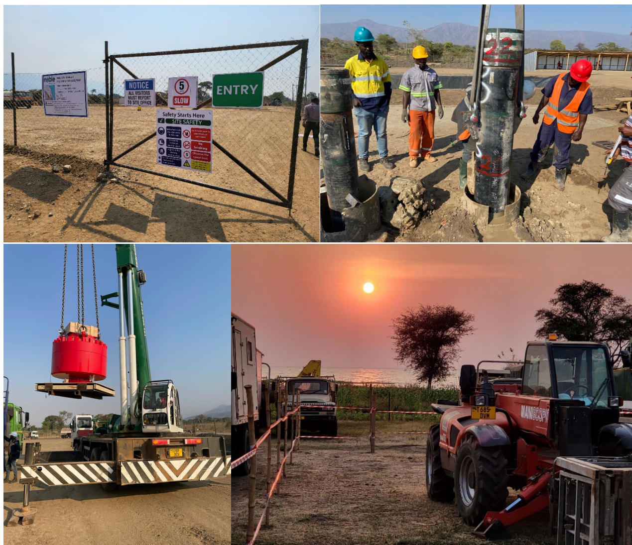
Figure 1. Clockwise from top left: Mbelele-1 site entry – safety first; installation of Mbelele-1 surface conductor; Mbelele-1 wellhead unloading; Drilling Camp sunrise over Lake Rukwa
