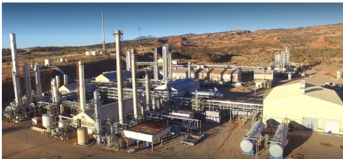
Figure 4: Paradox Resources "5.5 Nines" Lisbon Valley Gas Processing Plant.
