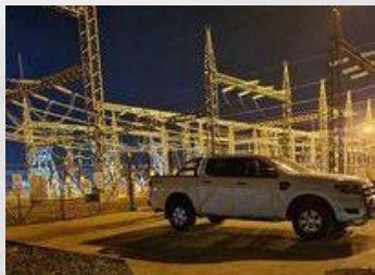
Eskom Substation 12km away
