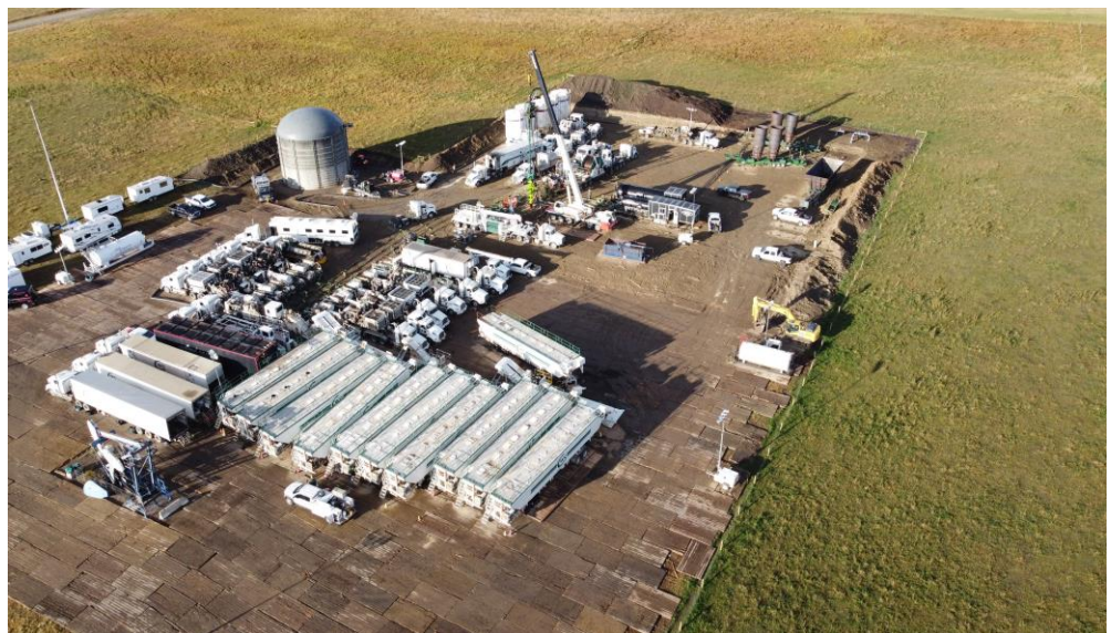
Figure1: Areal view of frac spread on location at the Certus Carol 1-27-33-05W5 well.
