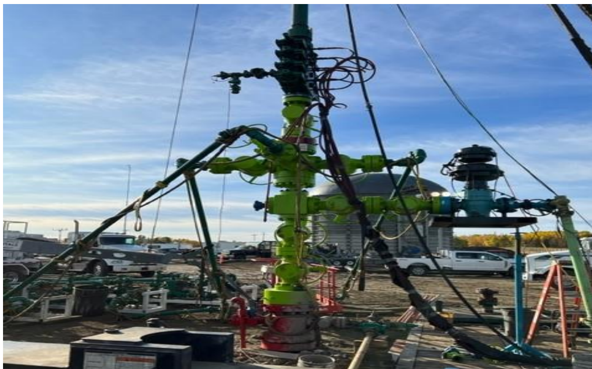
Figure 3. Certus Caroline Wellhead and Completion Frack Equipment on location.
